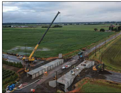
An aerial view of the installation for Pepin Creek Fish Passage in Bellingham, WA.
