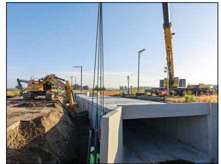
The main box culvert installation is complete, and outflow wing walls are being installed prior to backfill.
