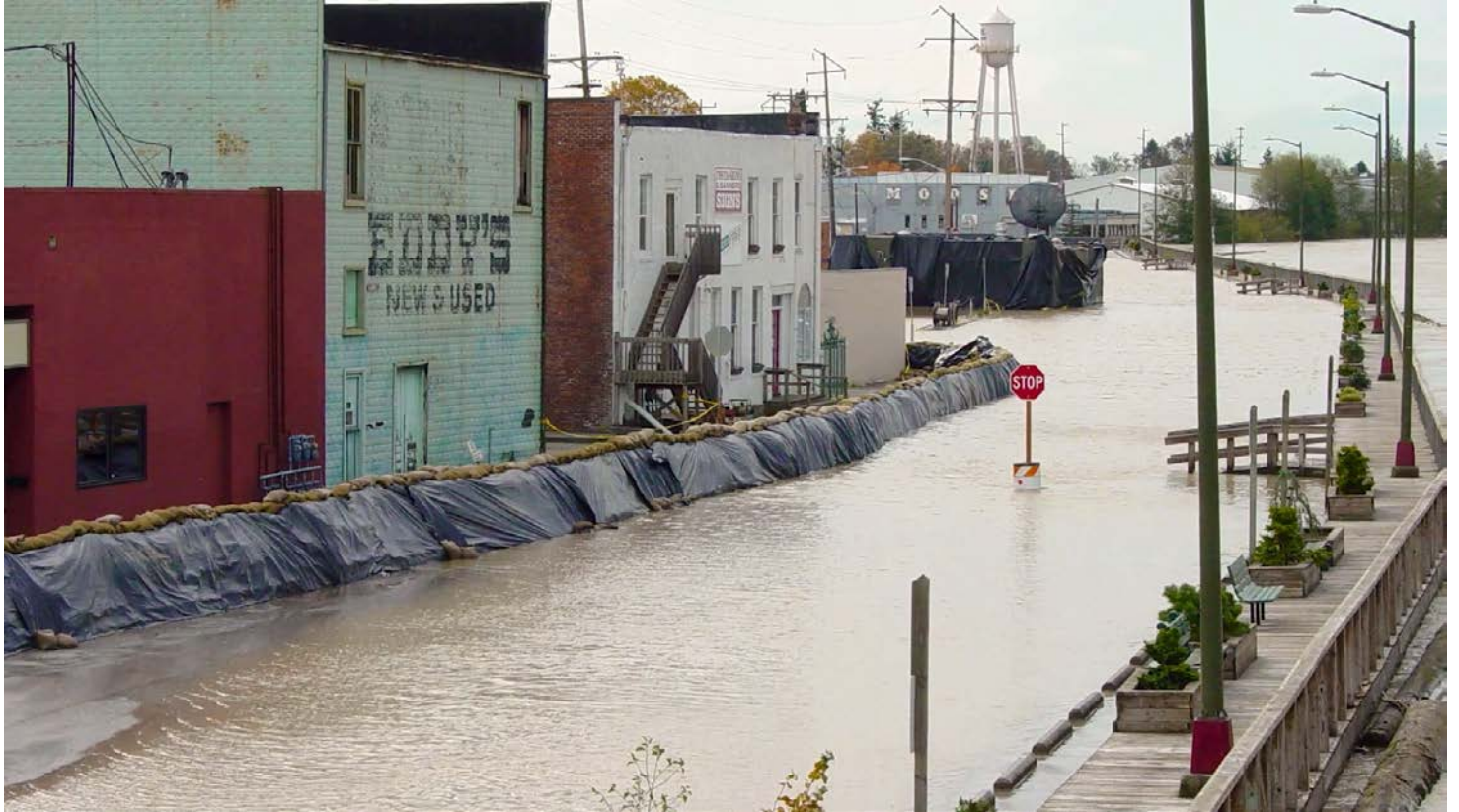
Top: A sandbag wall is built on Main St in downtown Mount Vernon by a crew of volunteers Bottom: Skagit River flooding on Main St prior to Floodwall installation
