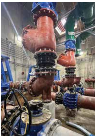
Underground valve vault containing the essential piping and valves for flow control.
